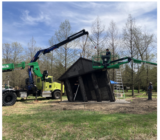
Installation of Ruins of Empire II or The Earth Swallows the Master's House at GFS
